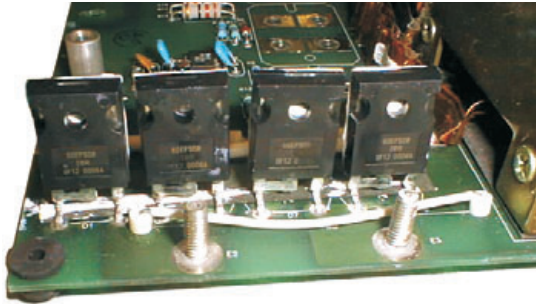
Figure 2.12. These four diodes need to be replaced.
